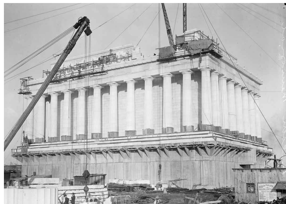
THE CONSTRUCTION OF THE LINCOLN MEMORIAL. COURTESY OF THE LIBRARY OF CONGRESS.
